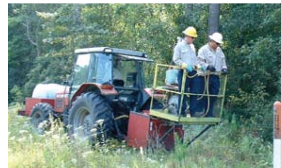
The cooperative uses both mechanical and chemical control methods to maintain right-of-way.
